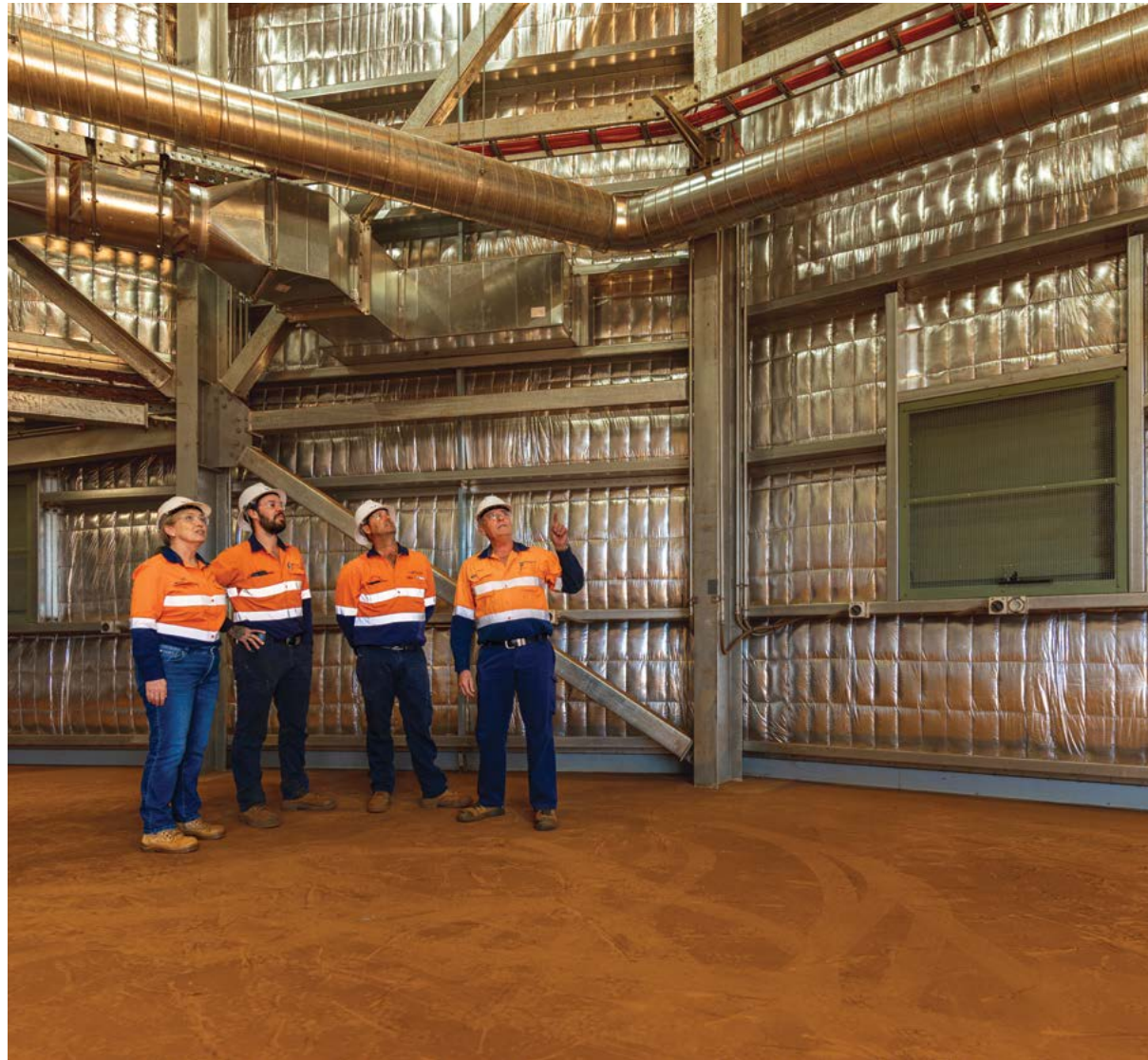
Administration Officer Sue Armstrong, Mechanical Supervisor Matthew Newett, Electrical Supervisor Chris O'Hara and Utah Landside Superintendent Stephen Myers inspecting a warehouse under construction.
