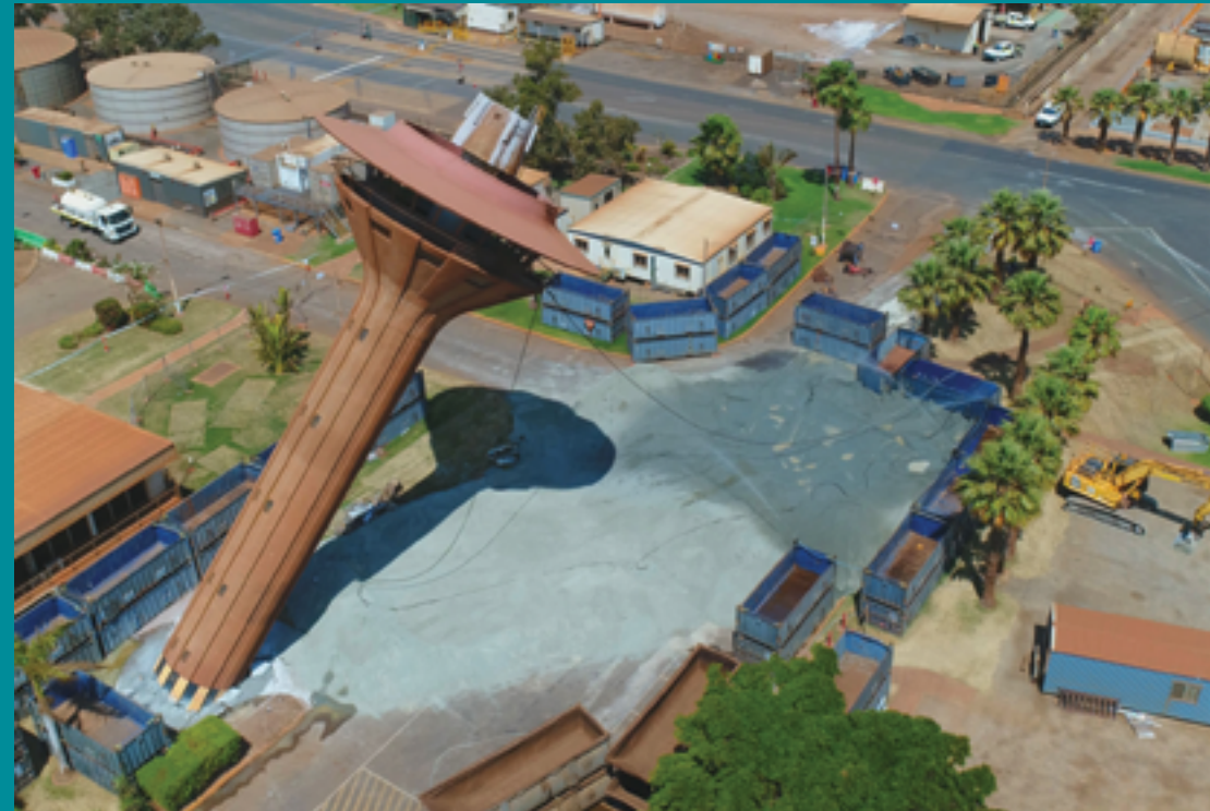
Felling of the Port Control Tower at the Port of Port Hedland
