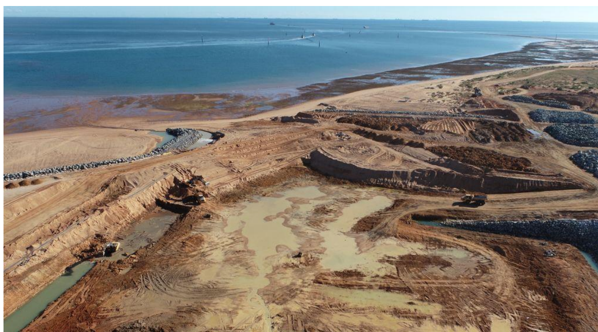
Figure 2: Construction works in the marina basin and inner rock revetments at the end of the Reporting Period, image facing north (July 2022).
