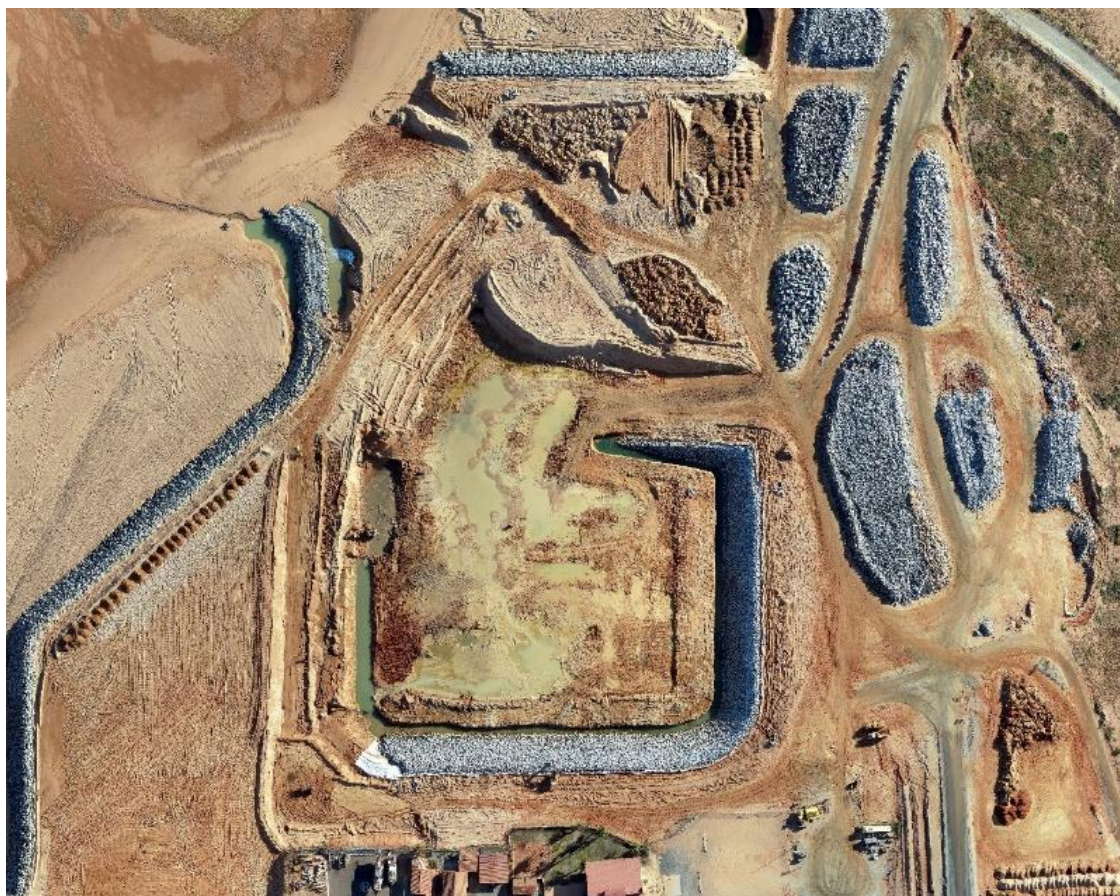
Figure 1: Aerial image showing excavations works in the marina basin, rock revetments and rock storage onsite at the end of the Reporting Period (July 2022).
