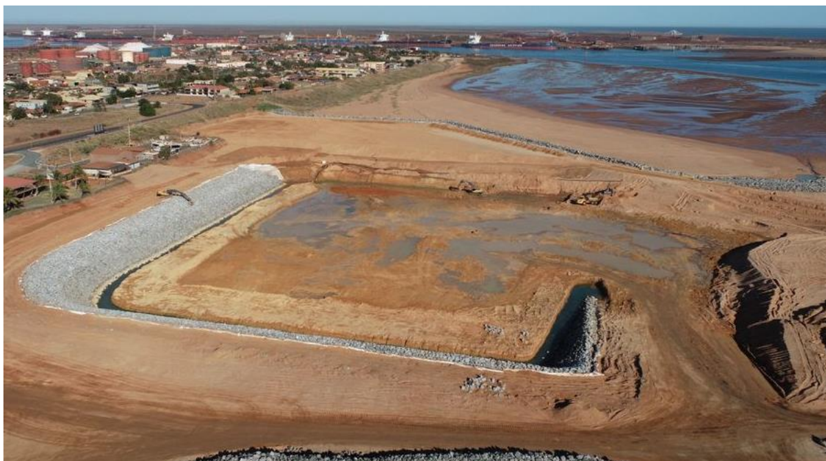
Figure 3: Construction progress of the rock revetment in the marina basin at the end of the Reporting Period, image facing west (July 2022).
