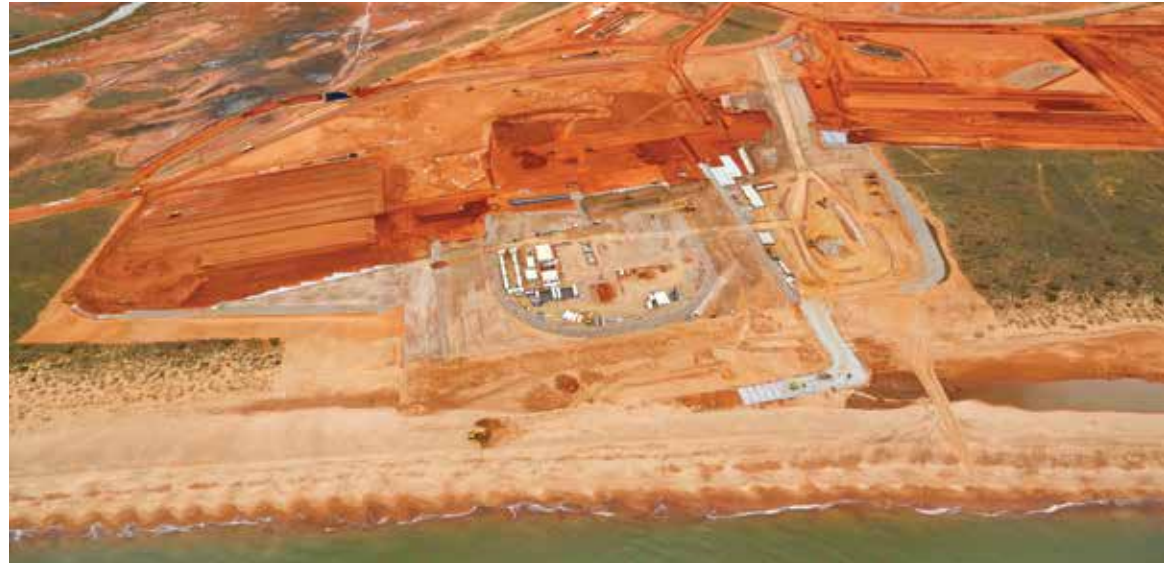
Port of Ashburton area early developments works of the Material Offloading Facility at the Chevron Wheatstone project (courtesy of Chevron Australia Pty Ltd)
