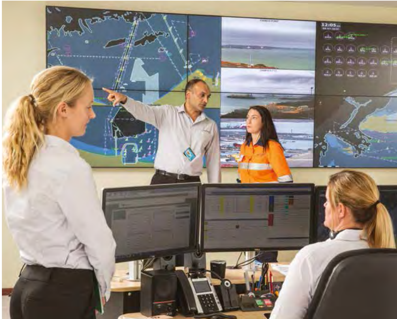
▲ Inside the Dampier Vessel Traffic Services Facility
